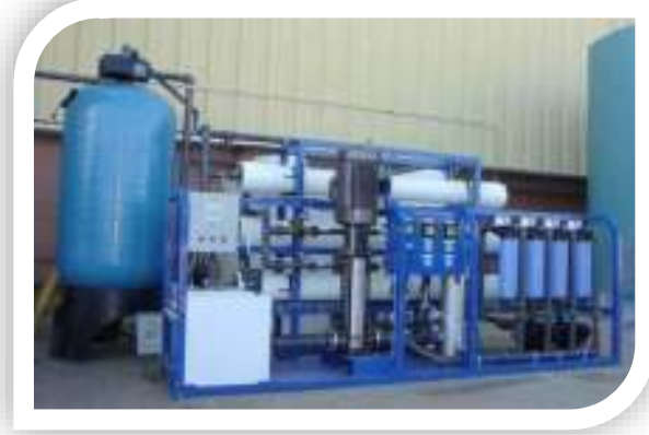
Water treatment units
